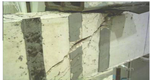
Fig. 18. Debonding and shear failures in group RS.
