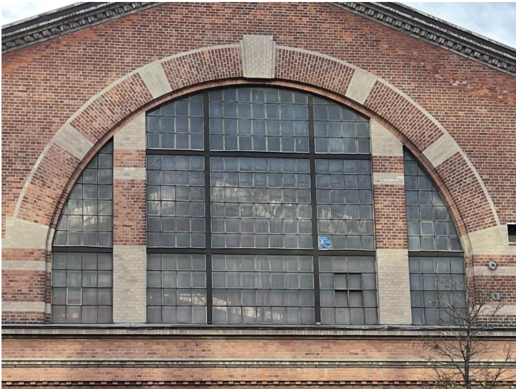
Figure 9 The large historic window on the south façade of the Machine and Assembly Hall, showing the segmented glazing arrangement with an upper arched portion and multiple rectangular panes. Photo by Varvstaden AB. Used with permission via email on 13 October 2025.
